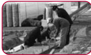
Volunteers are hard at work, as construction on the Habitat for Healthcare is underway.
